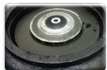
Compressor end oil leakage
