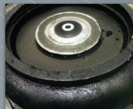
Compressor end oil leakage
